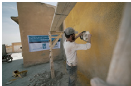
Rehabilitation of Najdat Al-salat school in Idlib after it was destroyed during the crisis.
